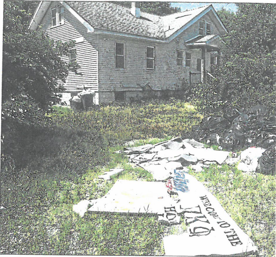
The exterior of the Pi Kappa Phi frat house in Egg Harbor City.
